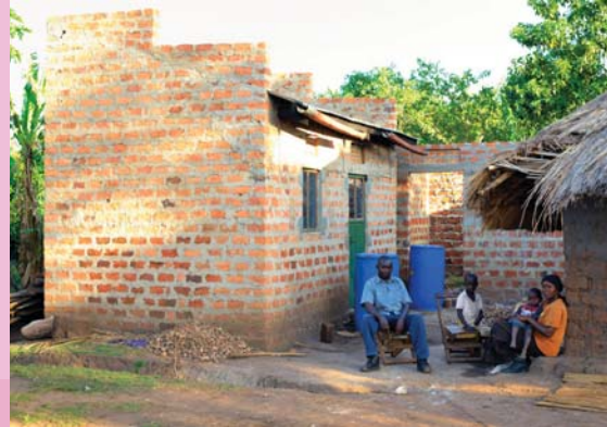
family sitting in front of their house which is under construction acquired through a loan support from ENCOT. ENCOT in partnership with SMF EA LTD
